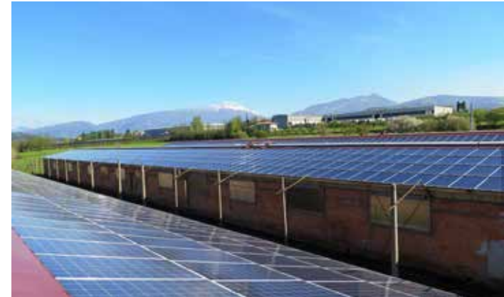
KPV in-roof system / Italy
